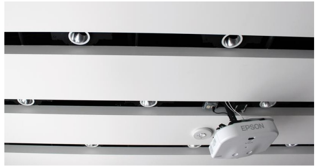
Figure 3: Recessed ceiling lights. Lights such as these are traditionally difficult to meter due to limited access to their wiring and uncertainty about the topology of the lighting circuit. Our Gecko sensors are easily and unobtrusively installed in fixtures such as these. See Figure 2(c) for a closeup view of the sensor mounting.
